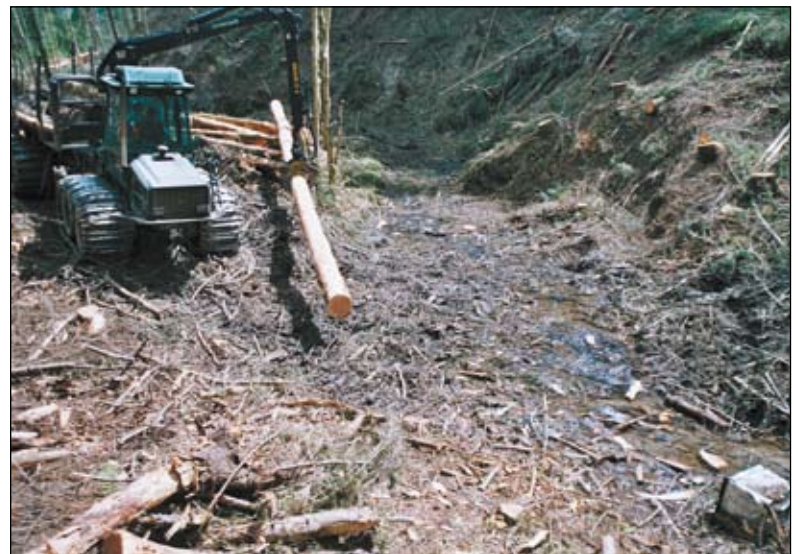
Barry Davies aboard the Timberjack starts to build another bridge across the water from a stock of timber set aside for the purpose. The harvesting operation had revealed the extent of fly-tipping to which the roadside woodland had been subjected. For example, a source of potentially dangerous contamination, in this case a discarded refrigerator, was found to be lying in the centre of the stream. It would need to be removed.
